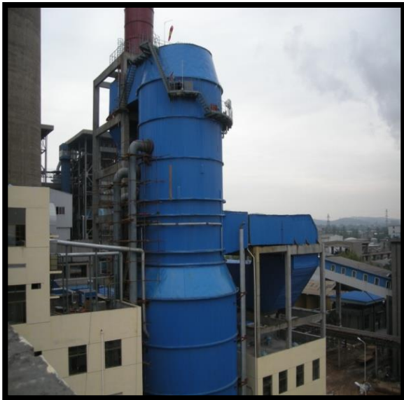
Qilu Thermal Plants Shandong Province, China
